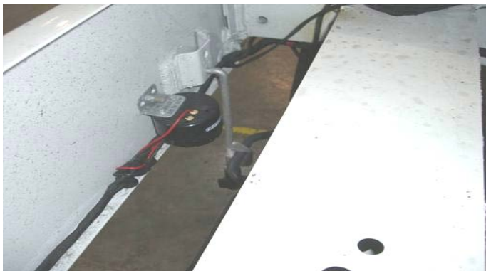
CODE JW0 - Alarm-rear backup, located at rear cross member
